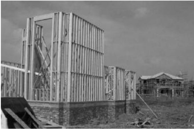
Members of the November technical and trade mission to China will visit wood frame projects in various stages of completion in Beijing.
