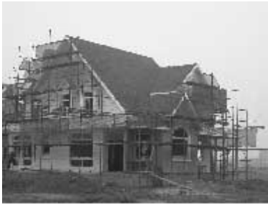
Wall systems by Premier Panels were installed in this model home duplex in the resort development of Kunshan.
