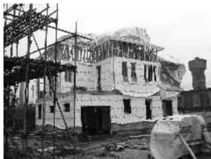
Engineered wood products and a range of materials from North America are used in the Dreamhouse project.
