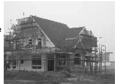
The use of SIPs in this duplex reduced installation time by almost three months compared to concrete.
